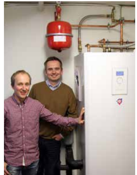
Kjell Ivar Kristiansen from SK Rør, installation company and Thor Erik Gjefsen home owner
